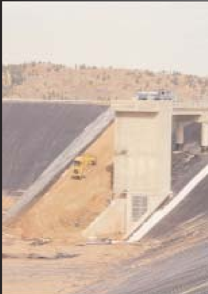
TESLA HYDROELECTRIC FACILITY - COLORADO SPRINGS, CO - 770,000 SF - 36MIL
